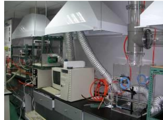
Local exhaust ventilation
