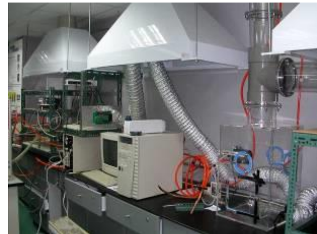
Local exhaust ventilation
